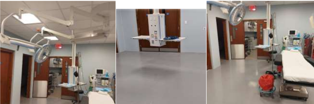
Operating Theatre – (Left and Right) Complete redesign and expansion with upgraded fixtures and equipment. (Center) Newly installed, state of the art MINDRAY Hyport 3000 Mechanical Pendant which offers great and new possibilities to the Operating Theatre.
